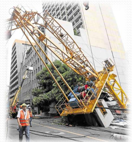
Tower crane collapse
