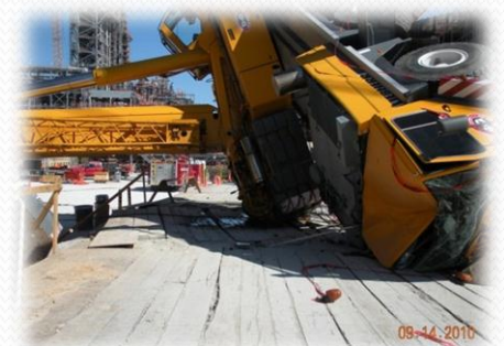
Mobile crane overturned
