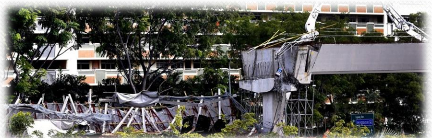
Collapse of bridge formwork during concrete pour
